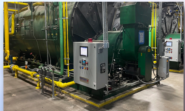
Photo 2: New natural gas lines and boiler controls installation at Manhattan Psychiatric Center
