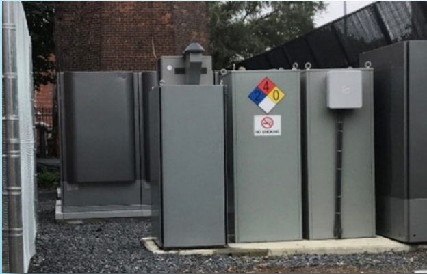
Photo 1: Fuel Cell Installation, Kingsboro Psychiatric Center
